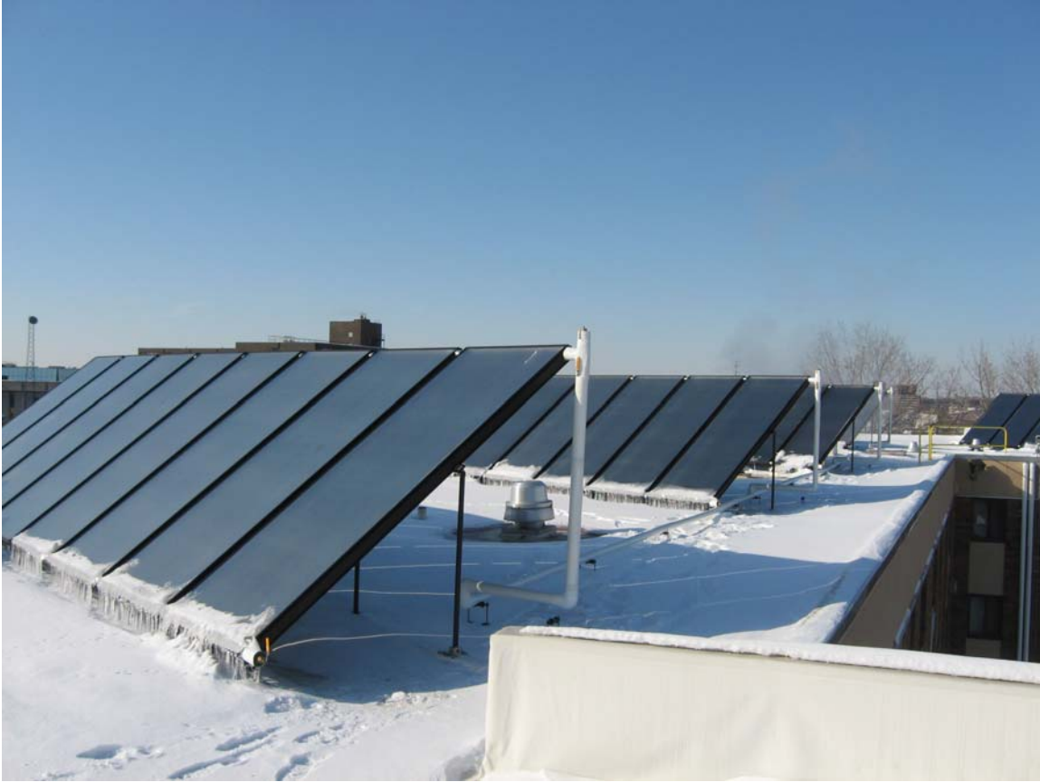
View of roof top solar collectors. Portions of 4 of the 6 arrays, each with 8 collectors are visible.
